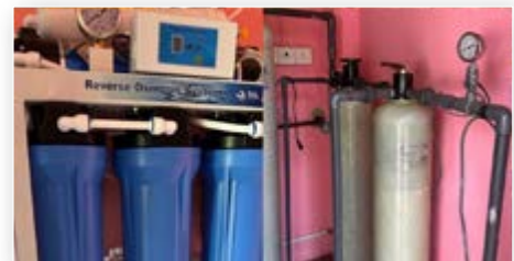
Installed a water purification project at Kapugollawa Maha Vidyalaya Horrawa Pathana to benefit 382 children.
