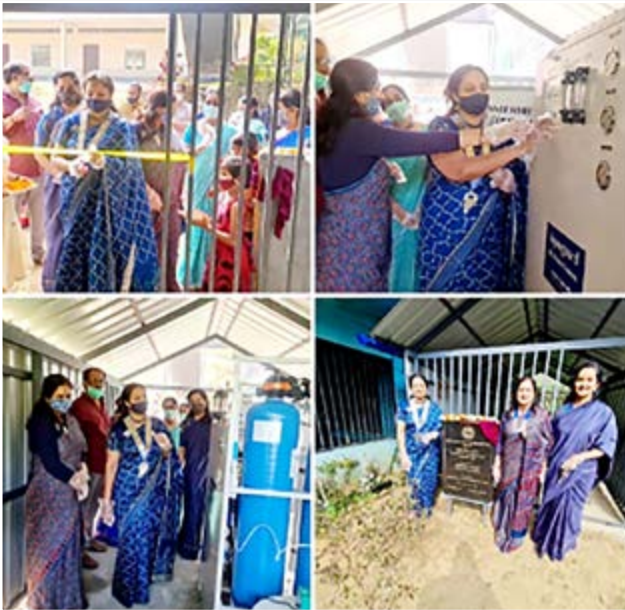
2020-2021. The Inner Wheel Club of Coimbatore West installed reverse osmosis plant for a tribal school in Coimbatore.
