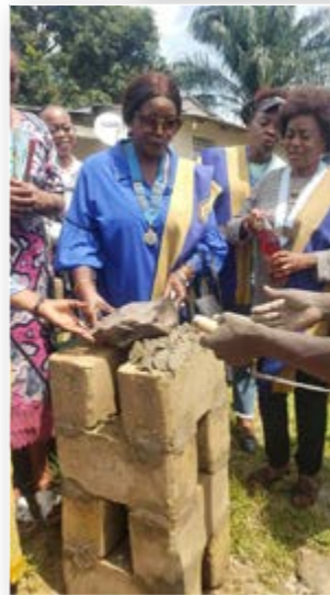
Laying the first foundation stones for a women's shelter in Fouban by the Inner Wheel Club of Kinshasa. (2023)
